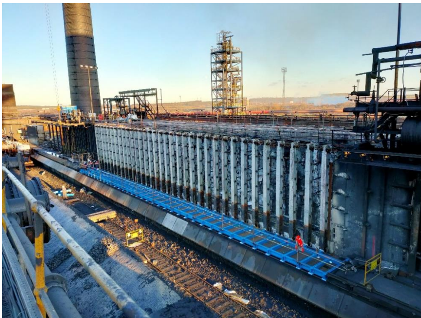
Figure 11: Battery 4 coke side steelwork and refractory refurbishment and the new gas collecting gas main being installed at Appleby Coke Ovens
