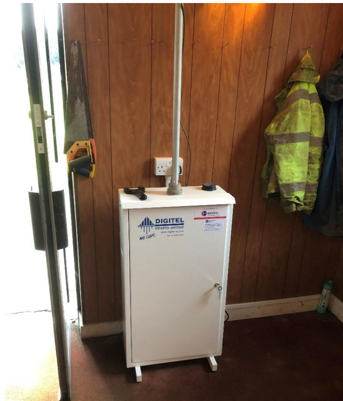
Image 1 The newly installed Digitel DPA14 sampler at the network monitoring site at Swansea Coedgwilym.
